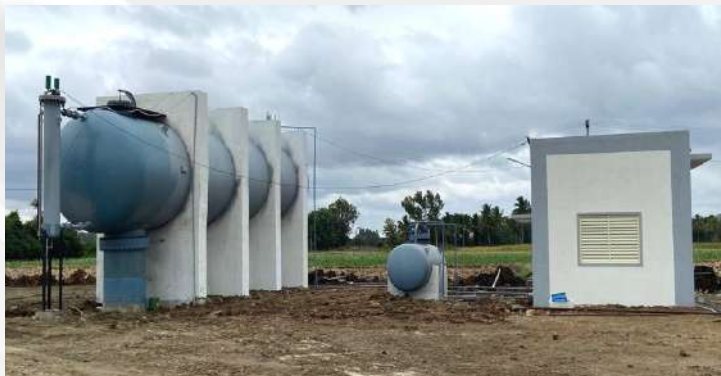
Conventional Type Surge Protection Systems
