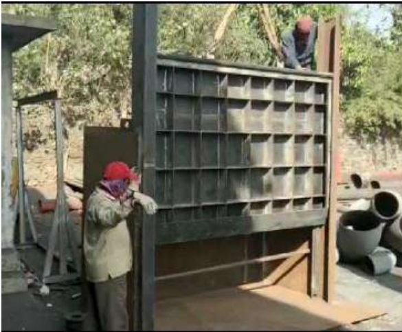
Stop Log Gates
