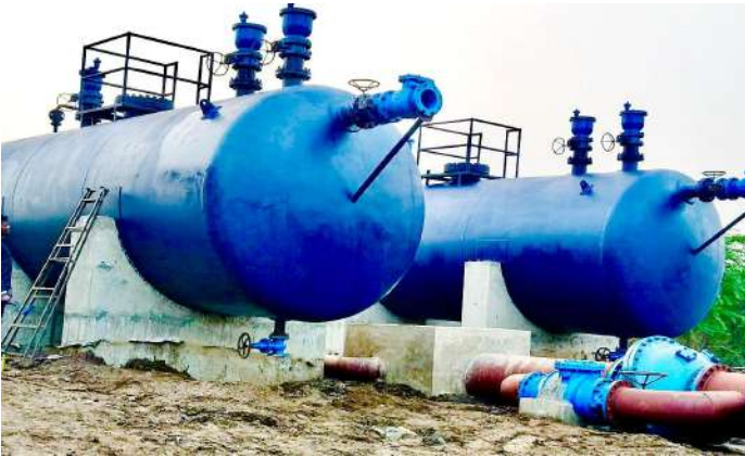
Two Way Surge Tanks
