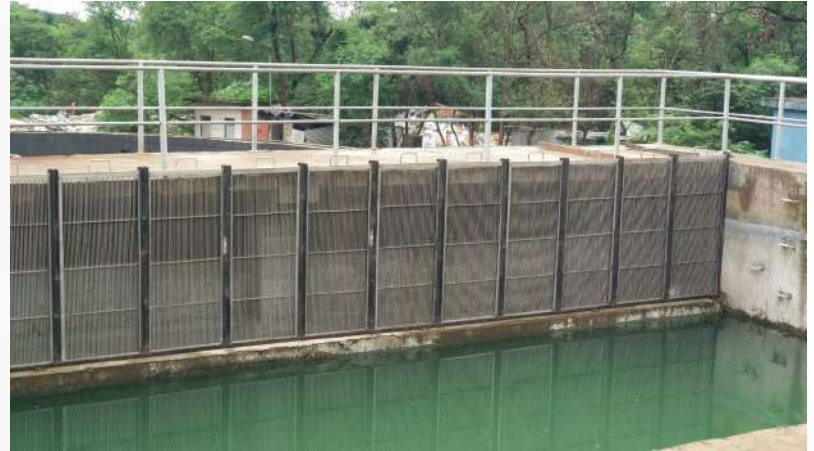
Trash Racks Fine Course Screens
